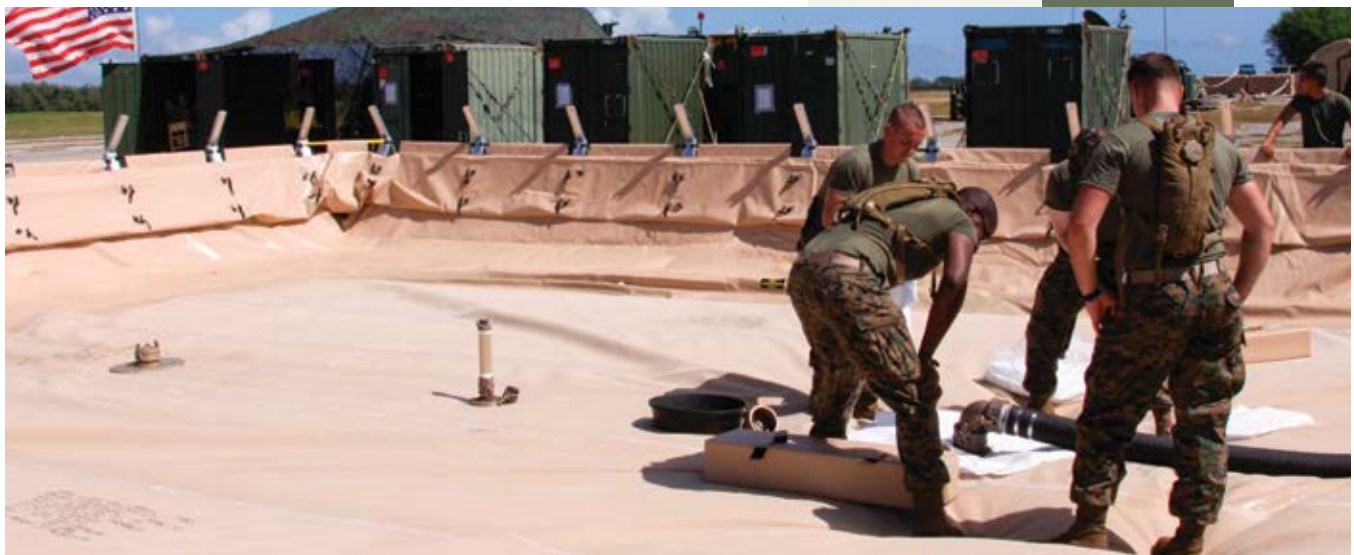
Fuel being transferred from a tanker to a storage bag with the All Terrain Berm™ providing secondary containment.
